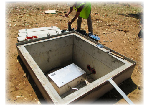
Rugged concrete vaults and heavy covering slabs protect installed instruments from the environment and vandalism.
